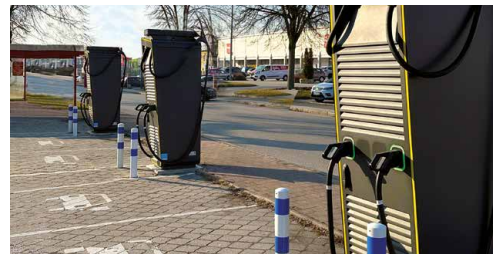
› Ladeinfrastruktur Eggenfelden 3 x DC Charging station, incl. transformer station
