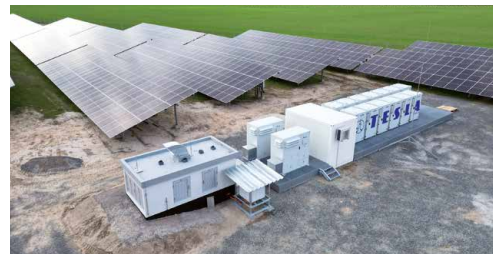
› Solarpark Rote Jahne approx. 6 MW incl. battery storage capacity with approx. 4,8 MWh
