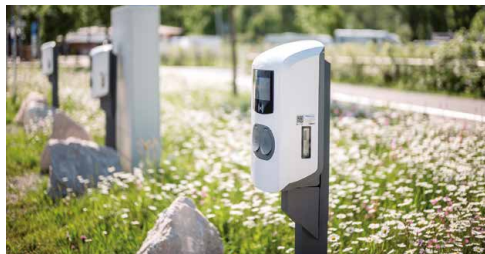
› Charging infrastructure Aschau im Chiemgau 1 x DC Charging station, 14 x AC Charging station
