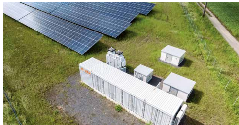
› Ground-mounted PV Reckertshausen approx. 10 MW incl. battery storage capacity with approx. 7,2 MWh
