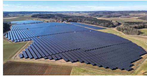
› Ground-mounted PV Amerdingen approx. 76 MW
