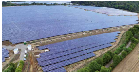
› Ground-mounted PV Niederelsungen-Wolfhagen approx. 97 MW
